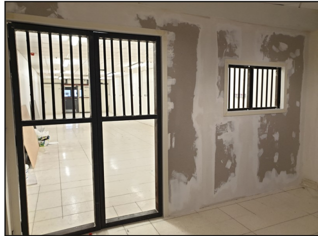
Figure 3: A strong room for potentially violent/criminal COVID-19 cases is also under construction. This used to be the hospital underground exit to the car park.
