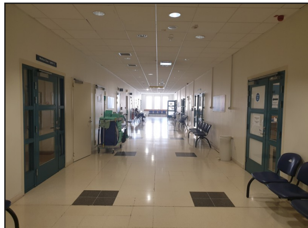
Figure 4b: This is an outpatient corridor and oxygen points can be seen snaking down from the ceilings.
